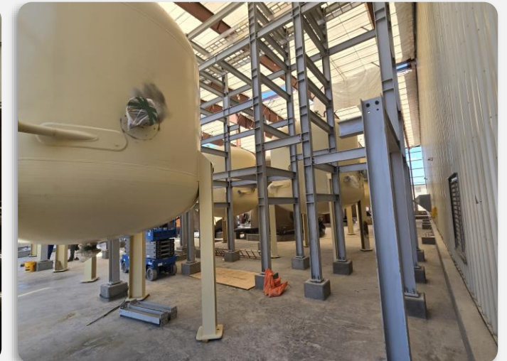
Ion exchange columns and pipe racks in new section of plant.
