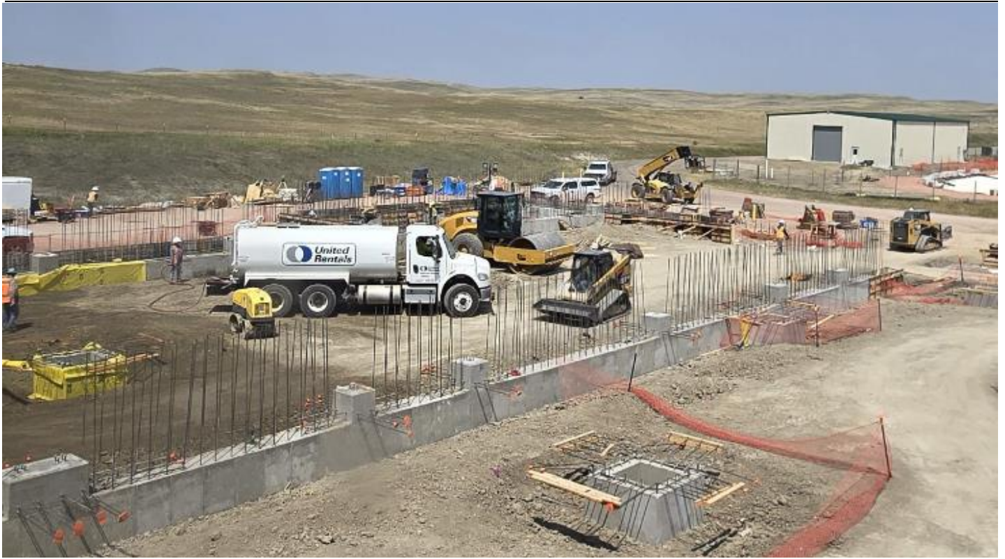
Figure 3: Crews installing forms in preparation for upcoming concrete pours at Ross CPP site
